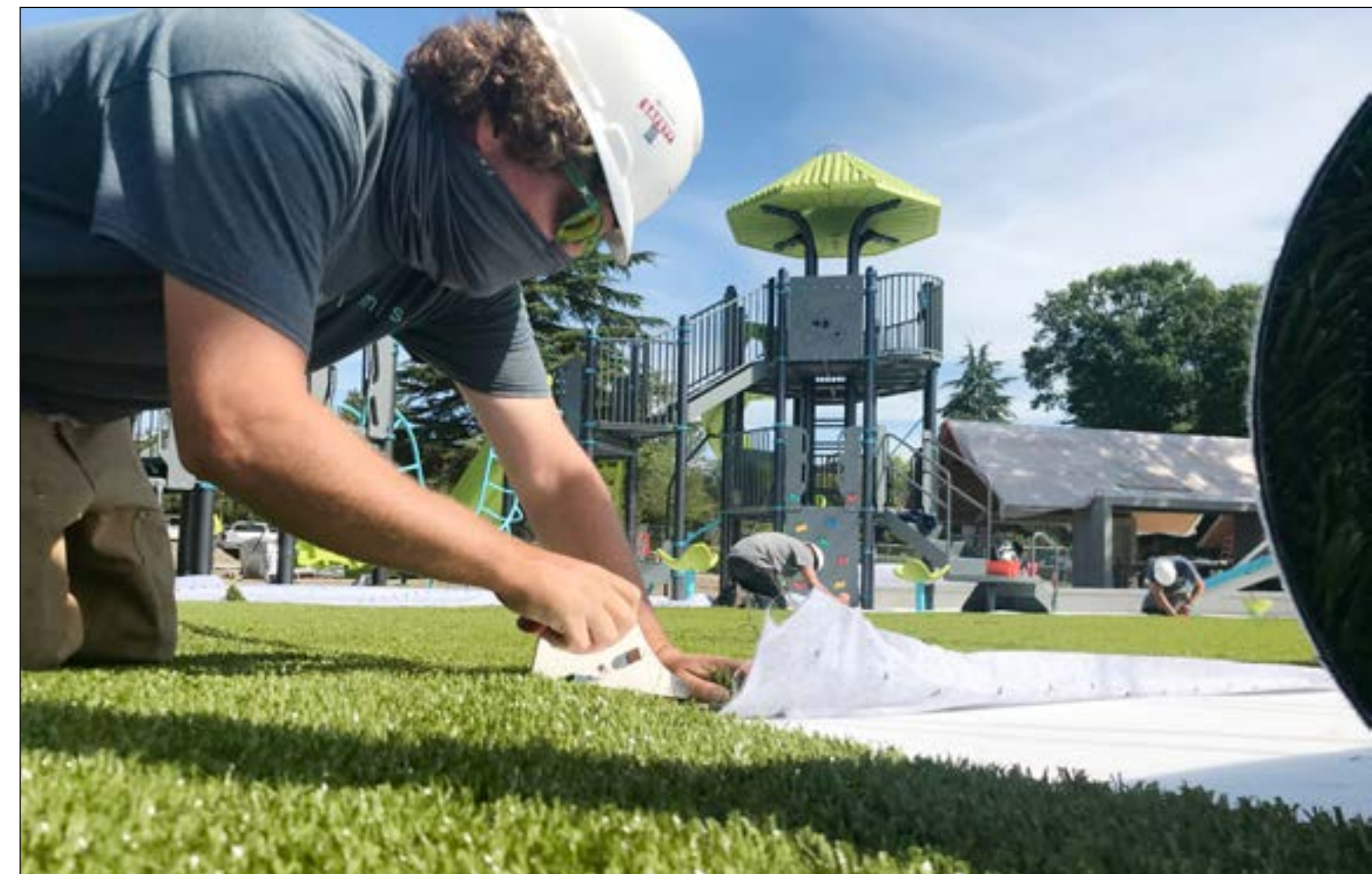
The City established guidelines to protect workers, who made progress on the park during COVID-19. Those guidelines included a COVID-19 safety inspector, face masks and closing the jobsite’s trailer to everyone, except the project’s two leads.
