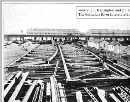
MANUFACTURING THE STEEL. View taken at Gary, Ill. All of the trusses were assembled at the shop, as shown lying on the ground here, all the holes for field rivets framed, and the different members match marked so they could be erected in Vancouver in just the same positions. This insured perfect matching of holes for the field rivets.
